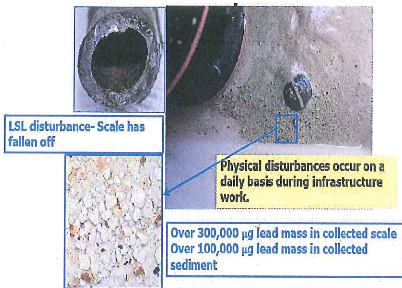
Figure 8: Significant Lead Can Be Released When LSLs are Disturbed
